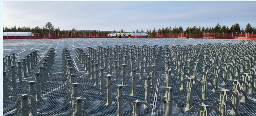
Partially installed antenna arrays (Kaaresuvanto, Finland)
